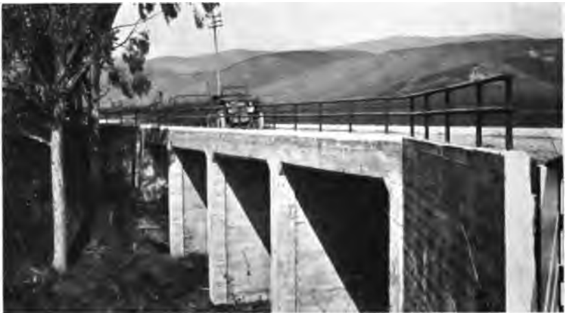
Near Half Moon Bay, showing type of guard rail used on bridges.
